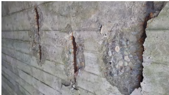
Fifth Avenue Culvert - Parging Recommended
