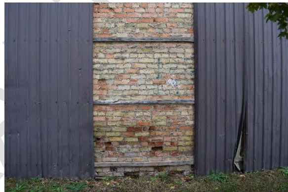
Plate 27: Missing corrugated metal revealing buff brick, looking east
